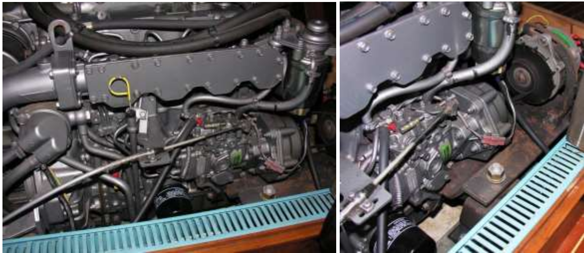
Starboard views note auxiliary generator
